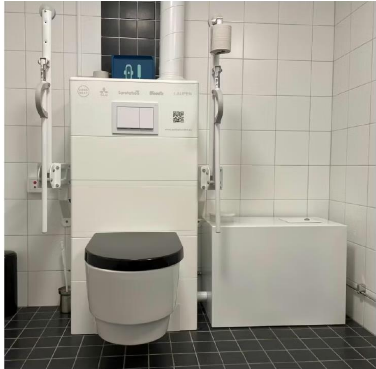
Prototype installed at VA SYD's HQ
